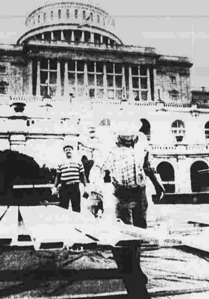
Inaugural preparations. Construction begins Friday on the West front of the Capitol in preparation for the presidential inauguration on Jan. 21, 1985.
